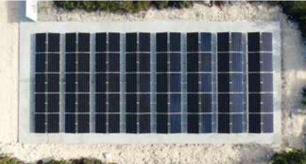
COMPACTGROUND, 32 kWp, Caribbean Islands
