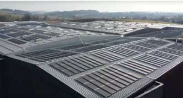
COMPACTMETAL, 1,236 kWp, Austria
