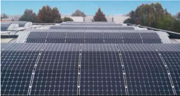
COMPACTMETAL, 80 kWp, Italy
