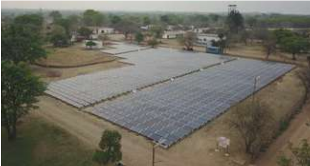
COMPACTGROUND, 500 kWp, Zimbabwe
