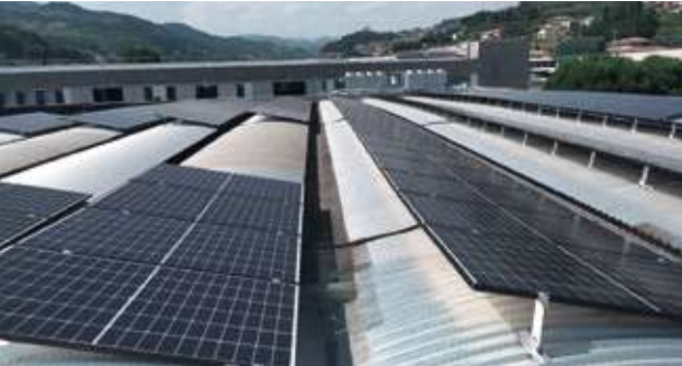
COMPACTFLAT, 120 kWp, Italy
